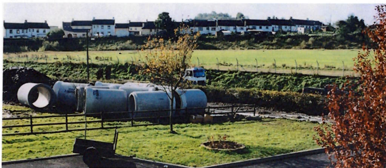
Railway road 2000/2001 - New pipes installed but floods continue to occur
