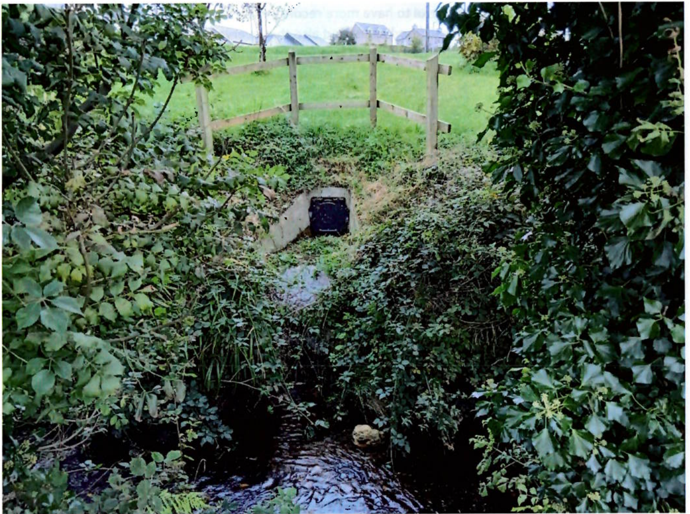
Blue stack park drainage into the current stream which regularly floods
